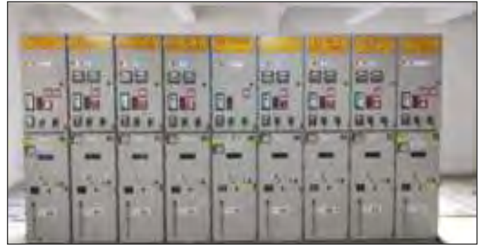
Indoor LT distribution panel
