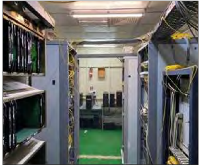
Server Room: South Campus
