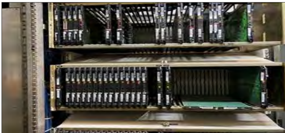
Telephone Exchange: Line Cards
