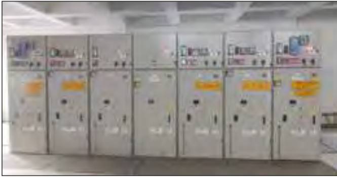
Indoor 11/0.415 kV (800 kVA) Transformer
