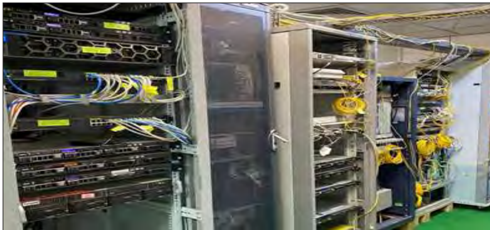
Switch Panel: Server Room
